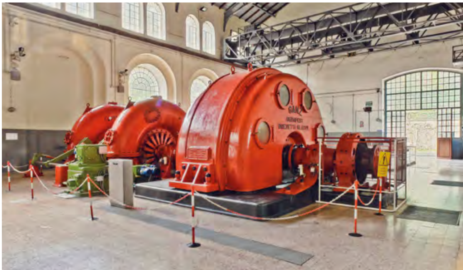
Castel Madama, Rome province, one of the turbines in the hydroelectric plant
